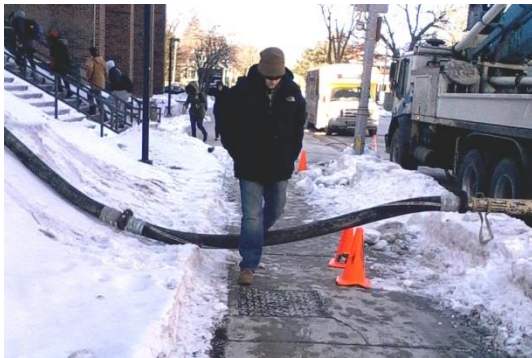
Figure 33. Concrete pump hose blocking sidewalk causing a tripping hazard.
