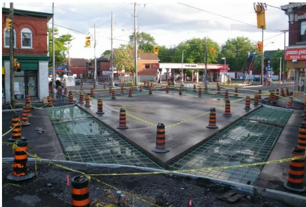
Figure 83. Concurrent construction of all four pedestrian crosswalks makes business access difficult (Canadian example). Note: Non-MUTCD compliant drums and improper closure of work site.
