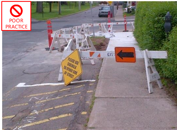
Figure 23. Pedestrians routed into live traffic lanes and non-compliant MUTCD sign.
