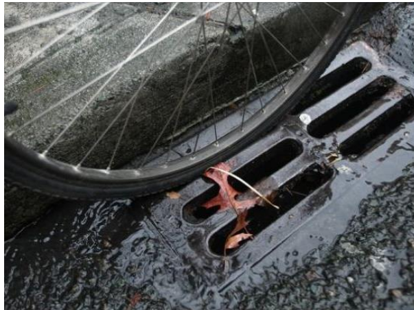
Figure 12. Some inlets are hazardous for bicycles.
