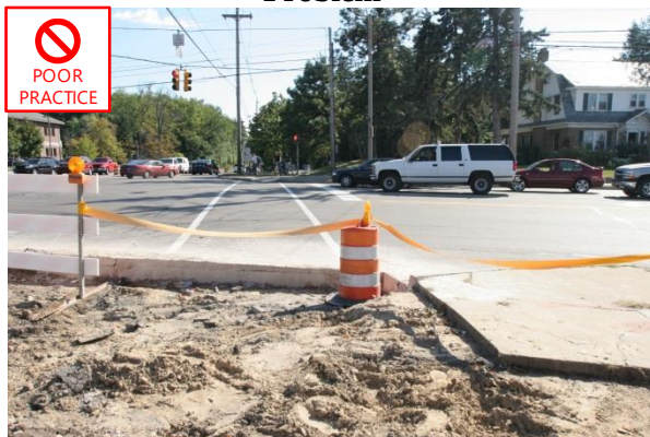
Figure 21. Pedestrians lead into closed area and inappropriate use of yellow tape.
