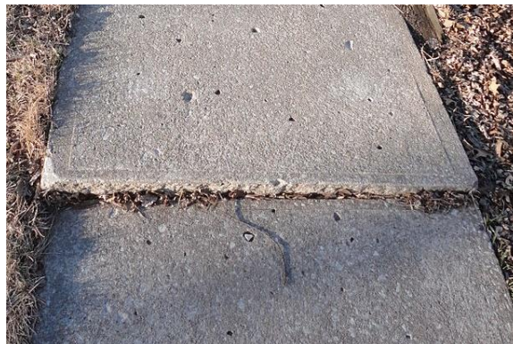
Figure 11. Existing sidewalk with vertical faulting. Source: Wikimedia Commons
