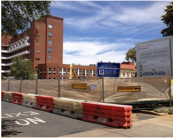
Figure 61. Separating pedestrians from urban street traffic using TL-1 crash tested plastic barrier system. Note: Non-compliant MUTCD color used for regulatory pedestrian sign. Source: Wikimedia Commons
