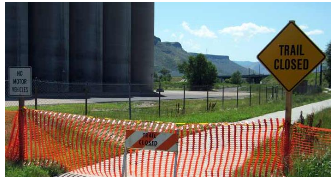
Figure 59. Orange plastic work zone fence used for closure. Note: Non-compliant barricade and sign on barricade.
