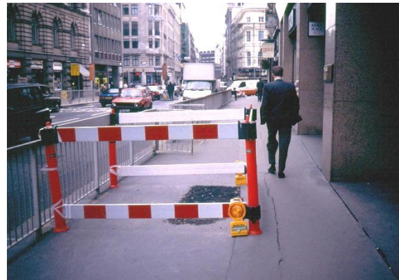
Figure 30. Barricade with ADA detectable bottom edge. Note: vertical stripes are non-MUTCD compliant. Stripes should slant toward the center.
