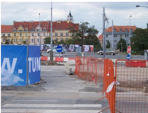
Figure 34. Potential tripping hazard from fence legs.
