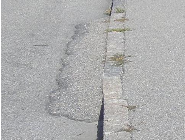
Figure 9. Raveling on thin edge of asphaltic wedge constructed without pavement milling. Source: UW-TOPS LAB
