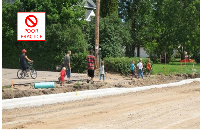
Figure 1. Pedestrians without appropriate fencing from a work area. Source: Wisconsin DOT
