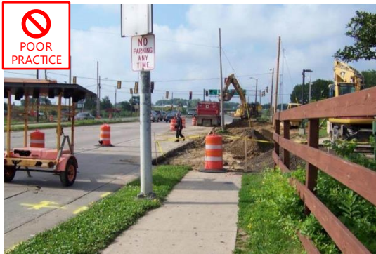
Figure 25. Non-detectable termination of sidewalk.
