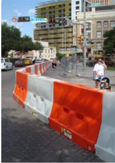
Figure 52. Orange and white longitudinal channelizing device/barricade used to separate pedestrians from motorized traffic.
