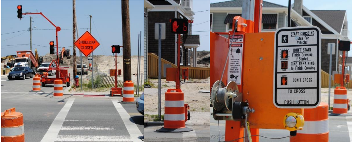
Figure 18. Temporary traffic signal with pedestrian signal indications. Source: Horizon Signal (IRF webinar)
