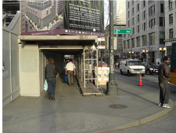
Figure 63. Falling debris protection at a building construction site. Source: City of Seattle
