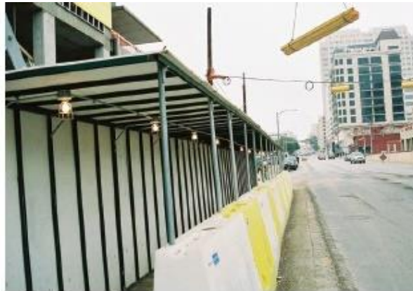
Figure 66. Reflector lamps instead of incandescent lamp bulbs could have been used to only direct light downward at this covered walkway.
