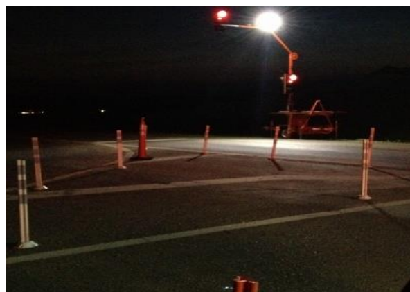
Figure 65. Light fixture mounted on temporary signal arm provides some crosswalk illumination, but glare partially obscures the signal indication.
