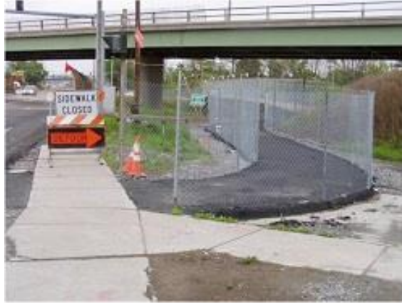
Figure 60. Semi-permanent chain link fence. Note: Need ADA detectable bottom rail on chain link fence. Source : pedbikesafe.org/PEDSAFE/casestudies/James M. Ercolano
