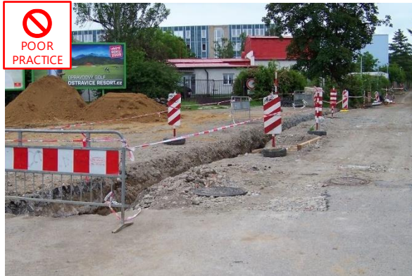
Figure 31. Trench delineated only by tape (Czech example).
