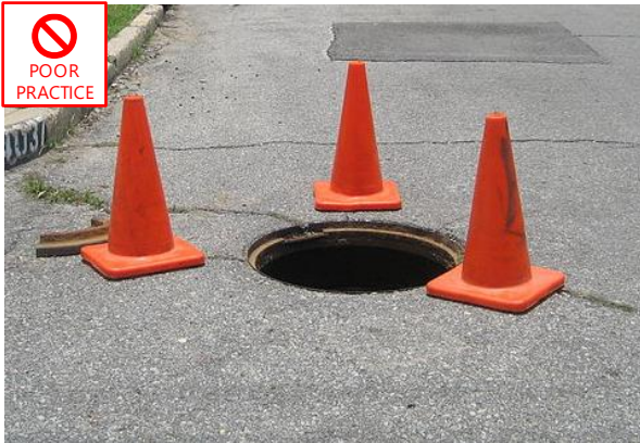
Figure 29. Open manhole (short duration). Not MUTCD compliant. Source: Wikimedia Commons
